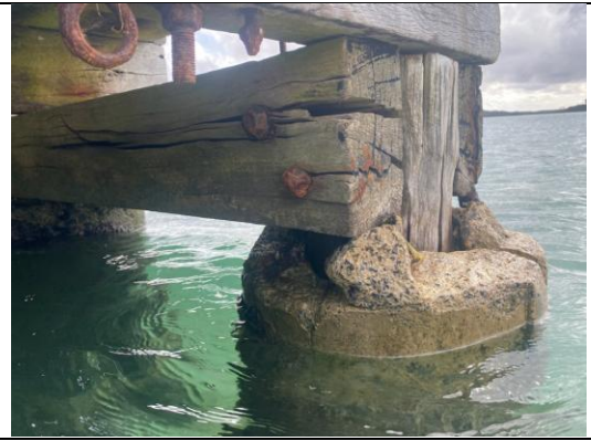
P6 Concrete Pot – extensive cracking & breakup
