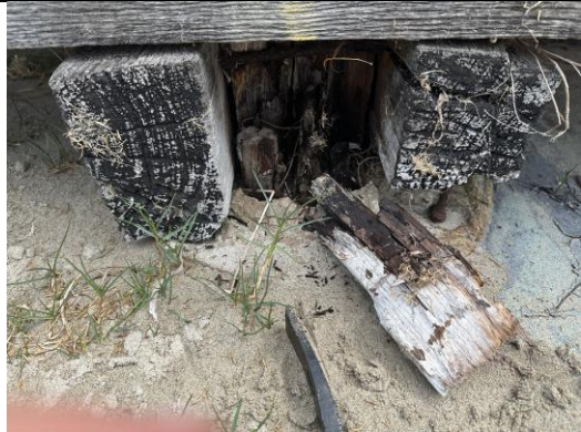
P7 Timber Pile – 30 to 40% loss in section due to rot
