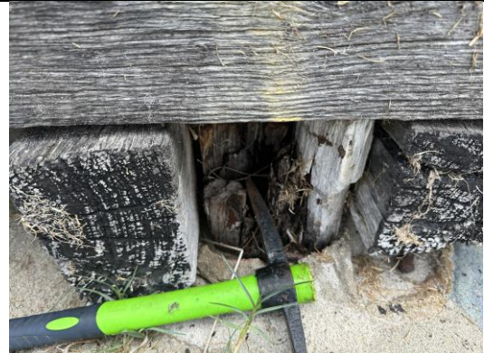
P8 Timber Pile – 30 to 40% loss in section due to rot
