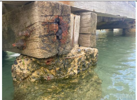
P2 Concrete Pot – extensive cracking & breakup
