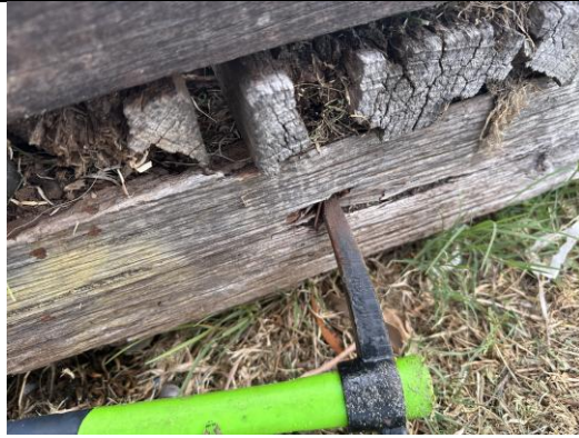
P11 Edge Bearer & Decking Ends – severely rotted
