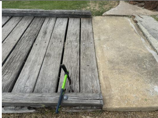
P15 Decking Planks – severely rotted
