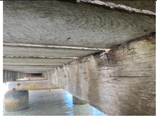
P12 Central Bearer – upper 30-50mm severely rotted
