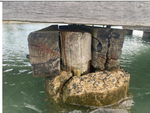
P1 Concrete Pot – extensive cracking & breakup
