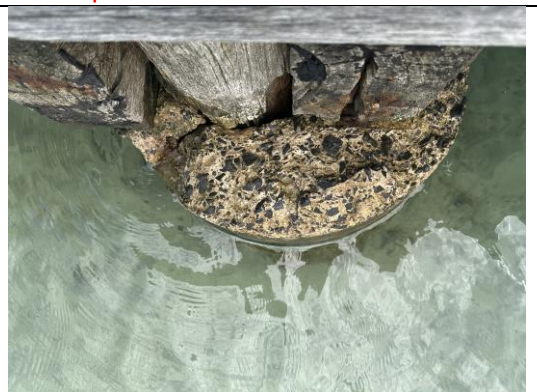
P4 Concrete Pot – extensive cracking & breakup
