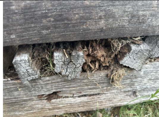
P14 Decking Planks – ends severely rotted
