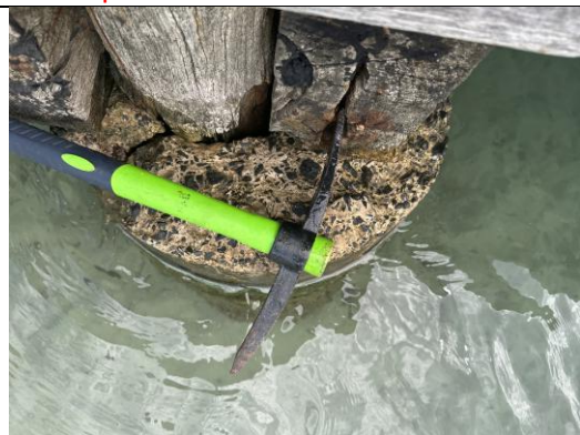
P3 Concrete Pot – extensive cracking & breakup
