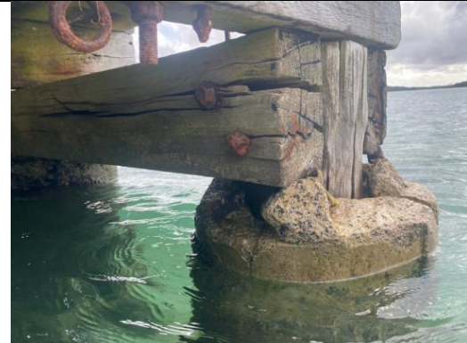
P11 Headstock – severe longitudinal split
