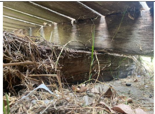
P10 Headstock – severely rotted
