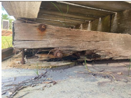
P9 Headstock – severely rotted
