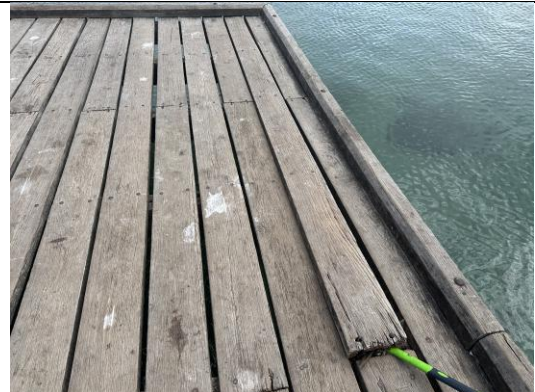
P16 Decking Planks – severely rotted
