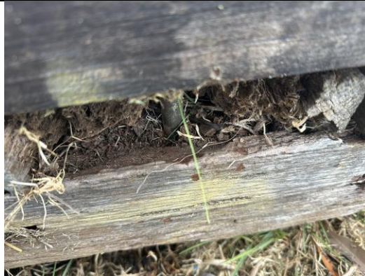
P13 Decking Planks – ends severely rotted
