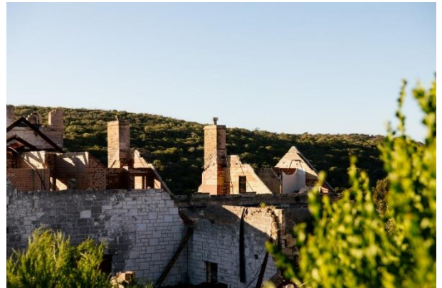
Figure 2-1 Image of the fire damaged Wallcliffe House. Source: Wallcliffe House Blog
