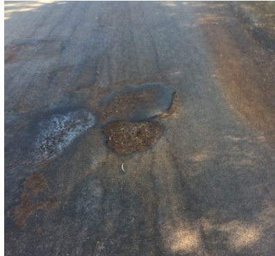
Potholes within existing roadway
