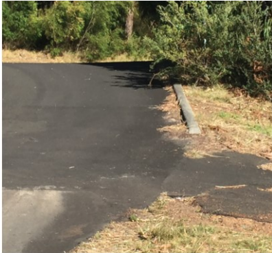
Edge break and general wear and tear evident within existing roadway
